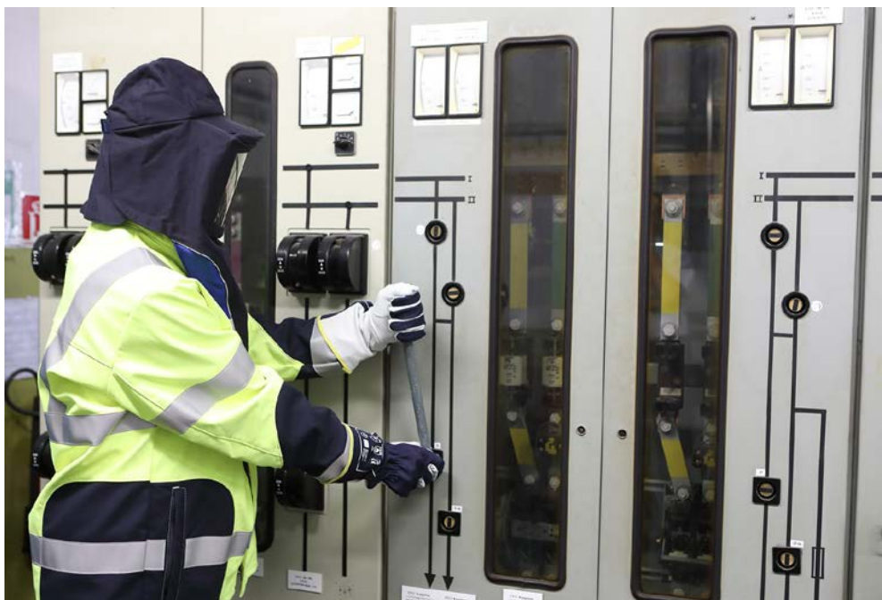
Fig. A 5-19 Opening the load break switch with a closed door by means of an operating lever
