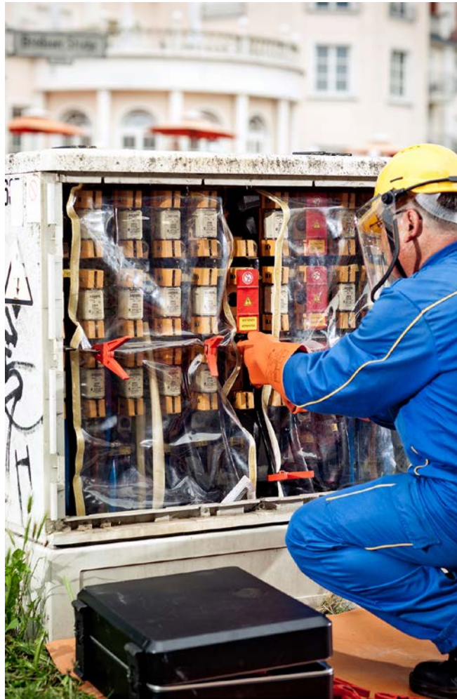
Fig. A 6-3 Working on a cable distribution cabinet: k_T = 1.5
