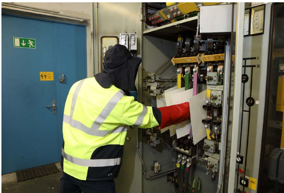
Fig. A 5-20 Removal of NH fuse-links, additional portable separators to isolate different potentials
