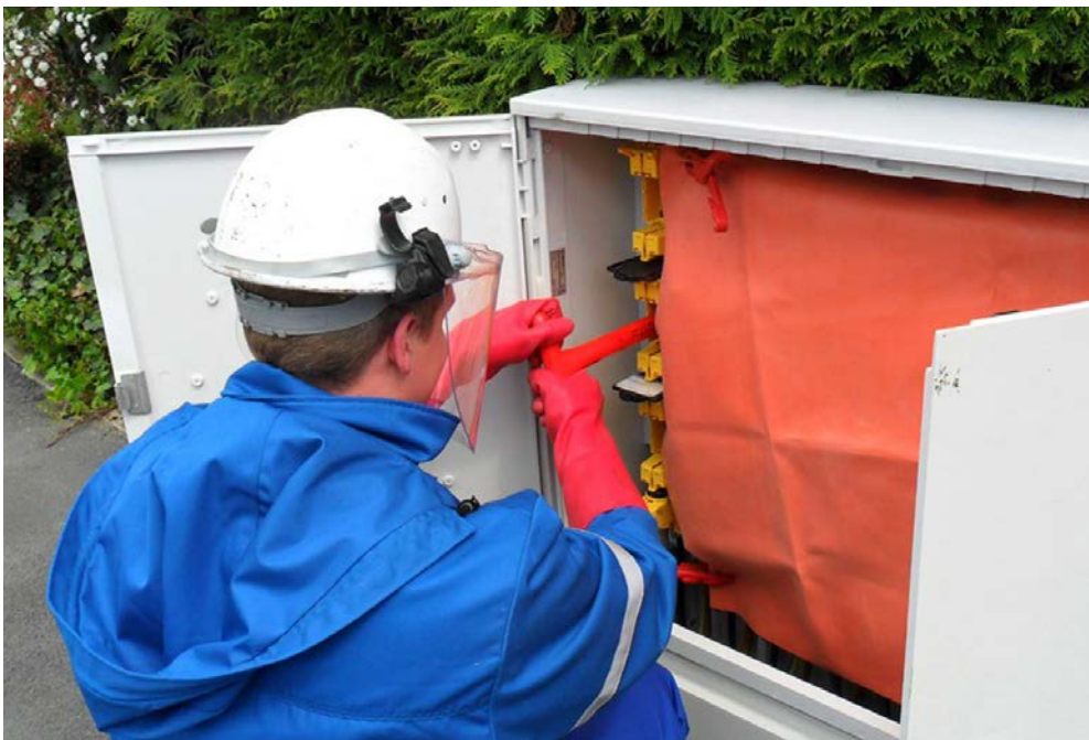
Fig. A 6-2 Replacement of a fuse panel in a control cabinet (close to the side wall): k_T = 1.0
